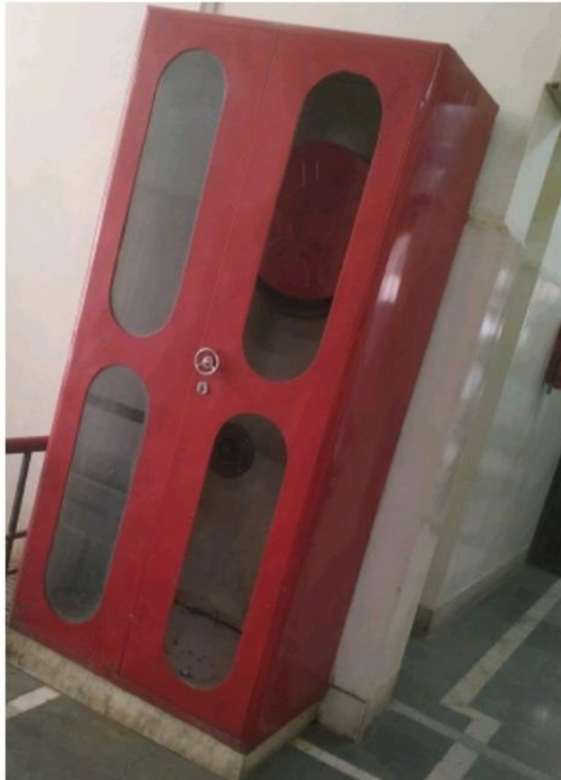
Figure.6. Internal Fire Fighting Equipment
