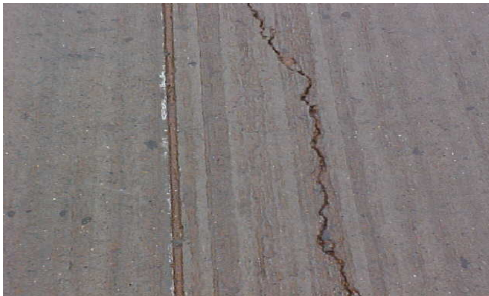
Photo 1. Transverse Crack due to Late Sawing
