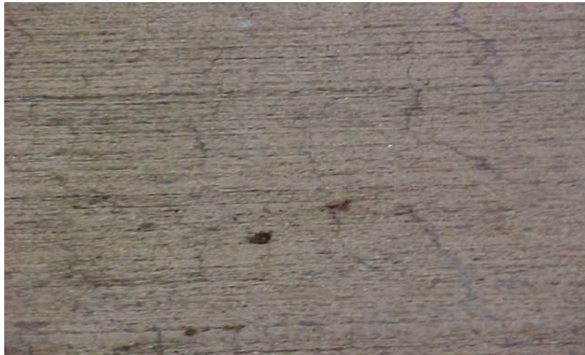
Photo 6. Plastic Shrinkage Cracks
